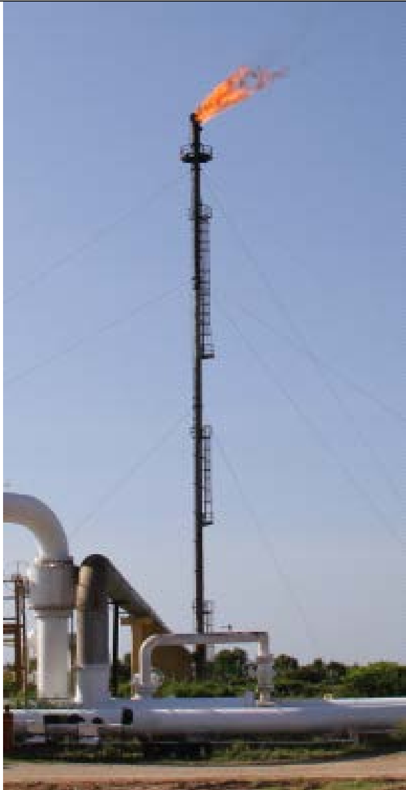
Figure 3: Photograph of Flare CCAC.7.19 at the CCAC.7 Compressor Station, 2, October 2014.
