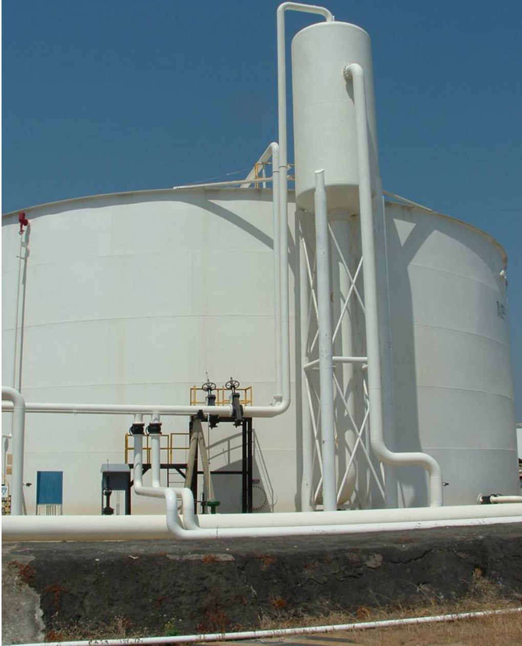
Figure 12: A photograph of a typical vapour recovery tower elevated above the storage tank.
