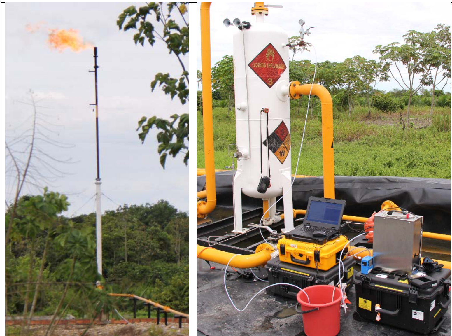
Figure 2: Photographs, from left to right, of the flare and flare knock-out drum with a tracer test in progress at Canuto Battery, 8 August 2015.
