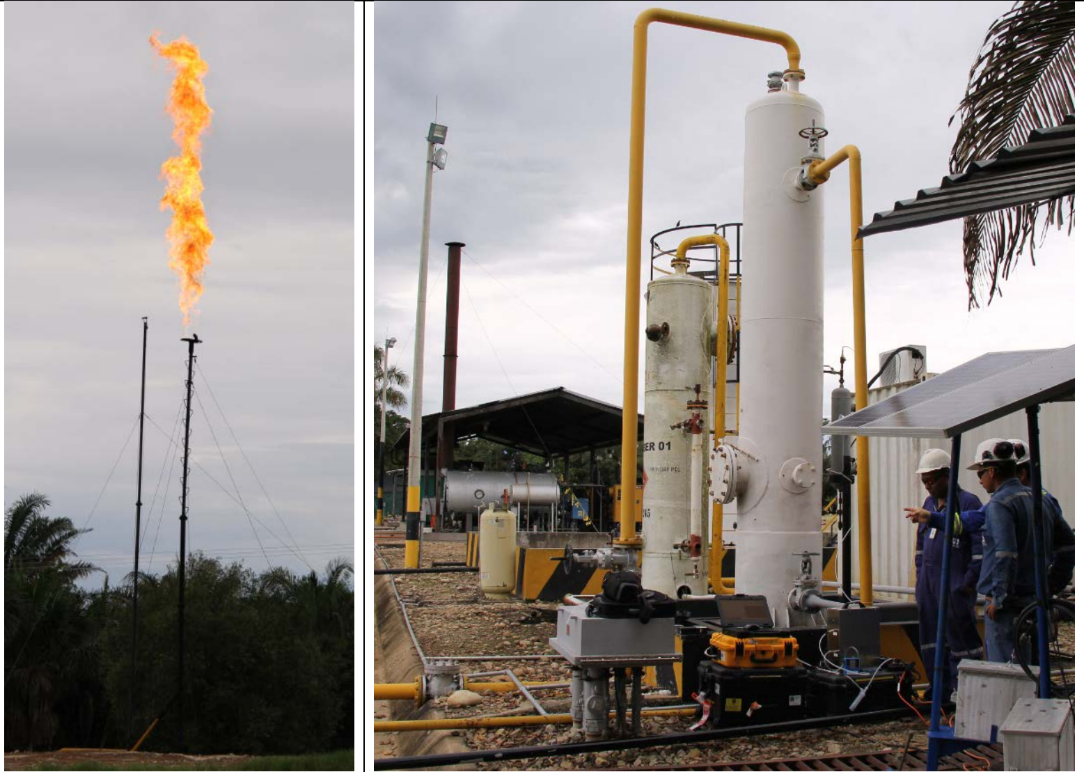
Figure 1: Photographs, from left to right, of the flare and flare knock-out drum with a tracer test in progress at CCAC.2 Battery, 9 August 2015.
