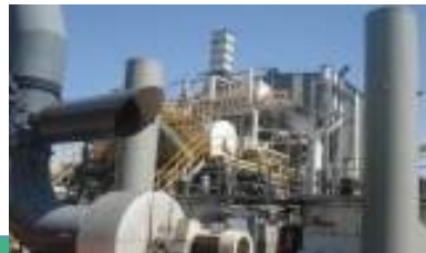
coal mine methane capture
