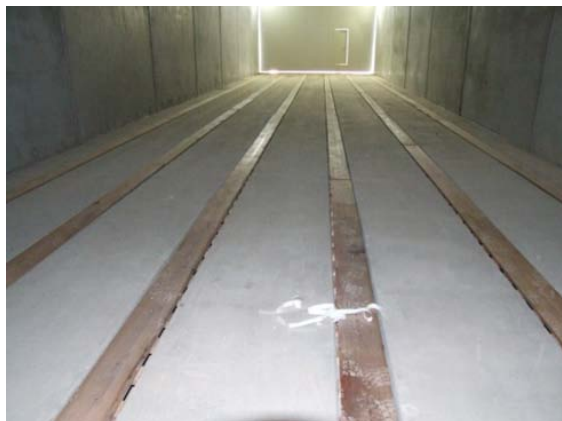
Inside a composting tunnel with aeration channels
