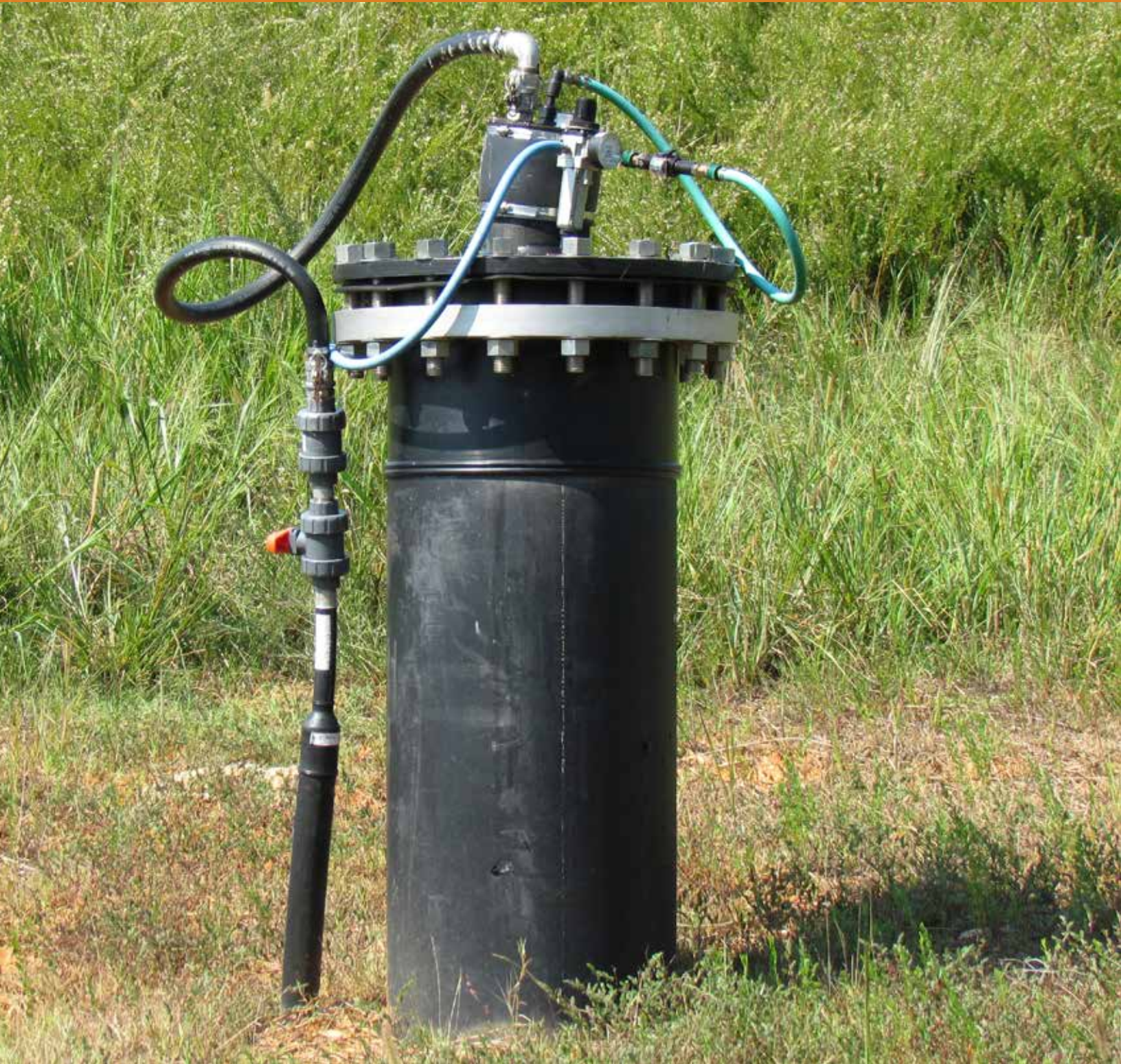
A condensate knockout pot and pumping system at the Orange County MSW landfill, North Carolina. If condensate is not removed, it can block the collection system and disrupt energy generation.
