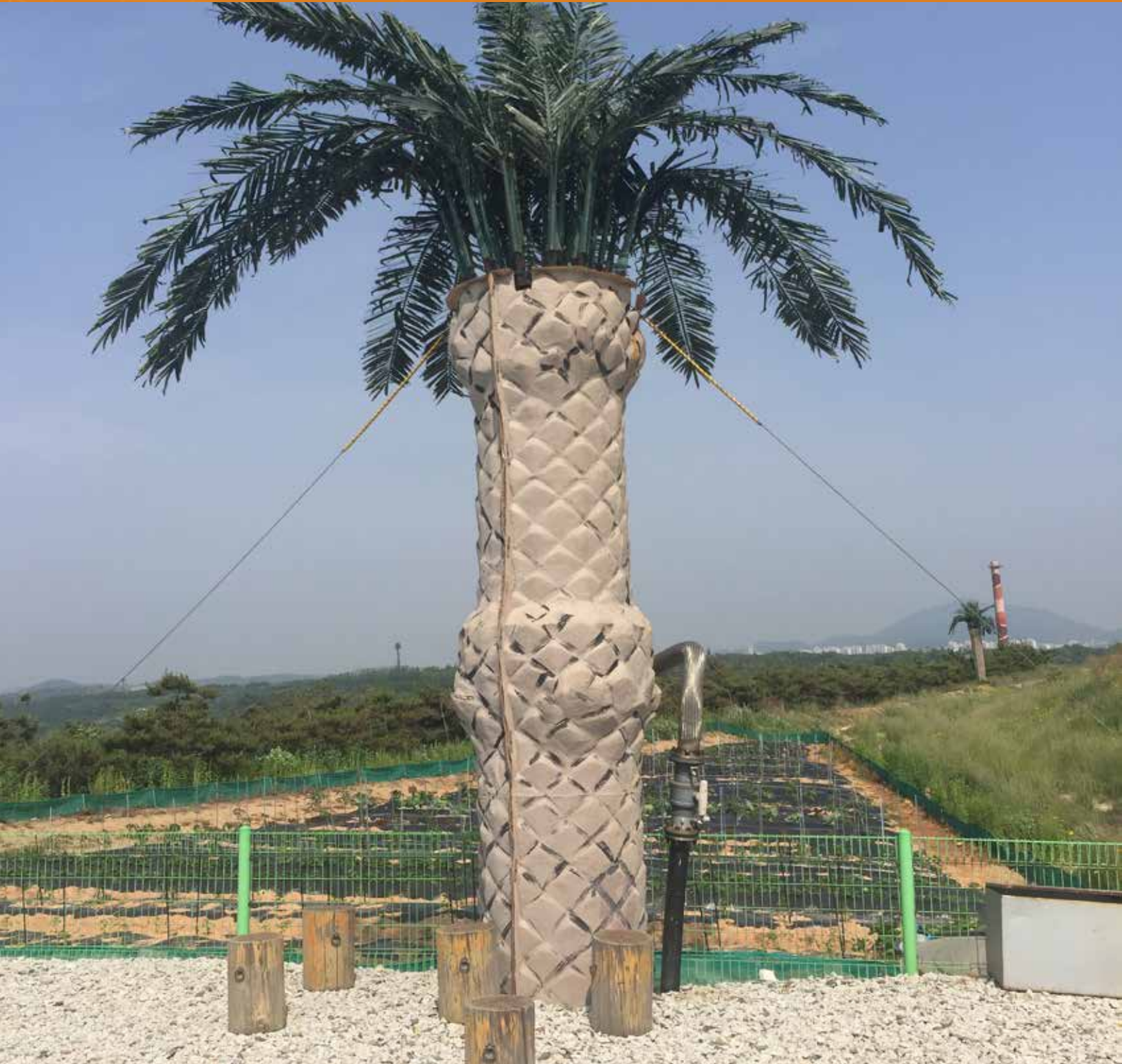
Landfill gas pipes aesthetically masked as palm trees at the Sudokwon landfill near Seoul, Korea.
