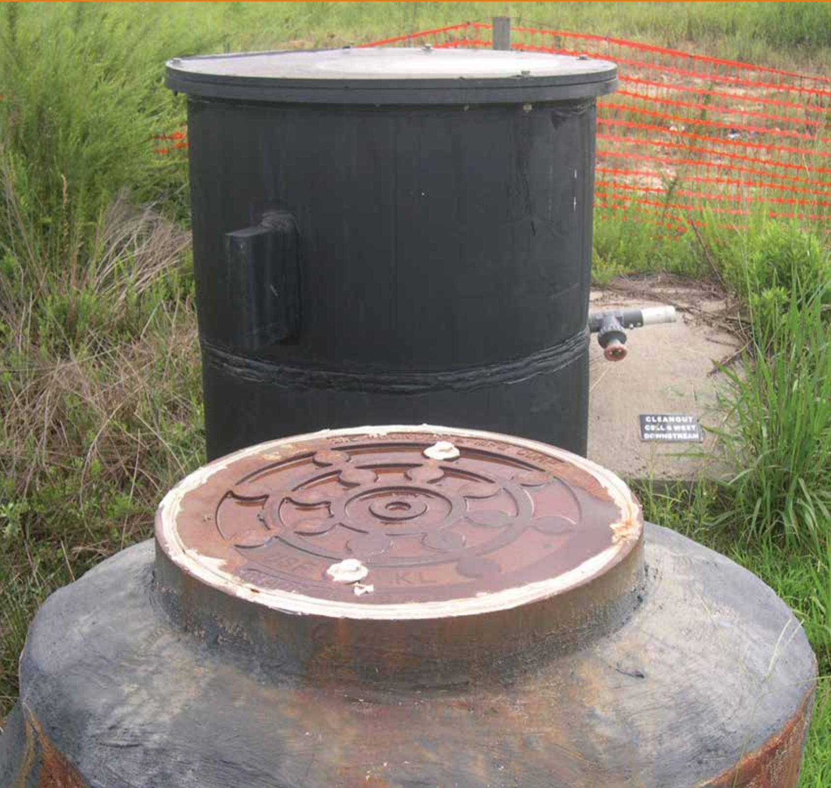
A leachate cleanout manhole at the Ann Street Landfill in Cumberland County, North Carolina. Regular maintenance of the leachate system is important for the success of a landfill gas project.
