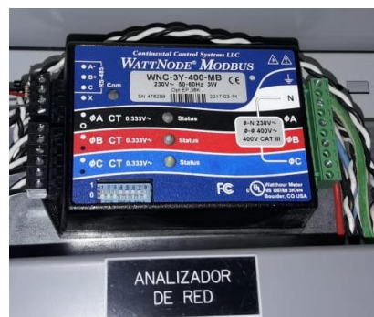
Figure 3.2. Picture of WattNode Gauge Installed at Tottus Alderete
