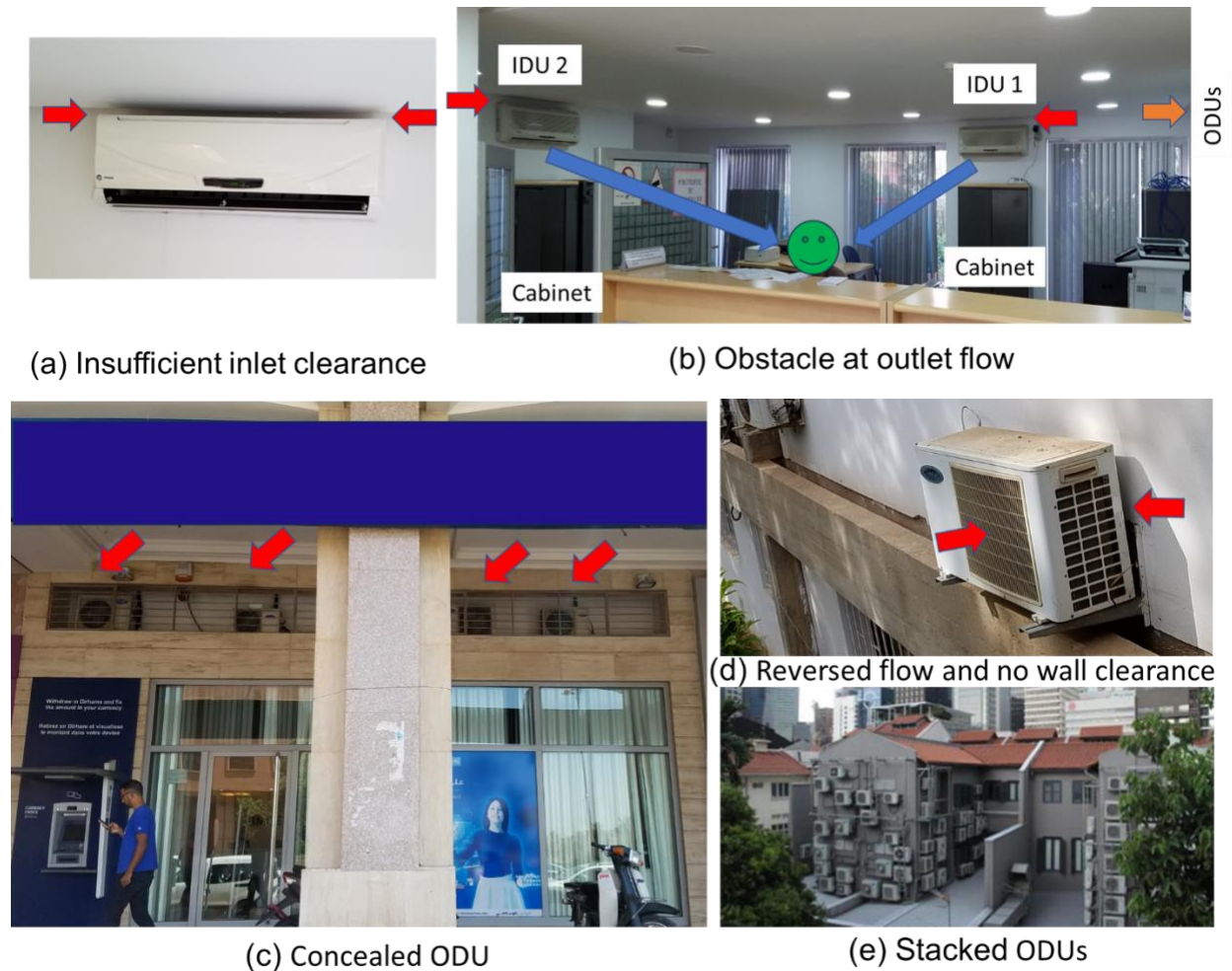
Figure 1: Poor installation examples.
